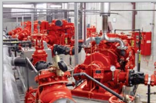
Horizontal Split Case Fire Pumps with diesel engines.
